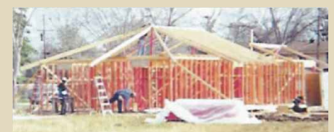
The first of four homes under construction in Lake Charles, Louisiana, with help from CHRISTUS and two lender partners.
